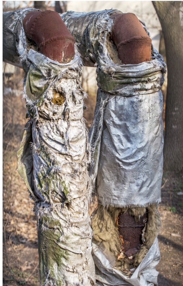
FIGURE 1. Damaged insulation is a major source of heat loss.
