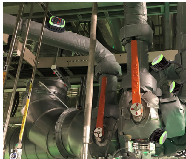
FIGURE 8. Components such as valves can be significant sources of heat loss and should be insulated
