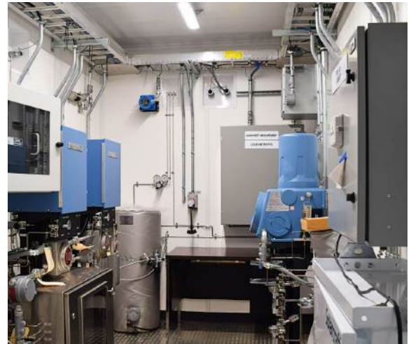
Analyzer Shelter with Gas Cylinder Warmer in use
