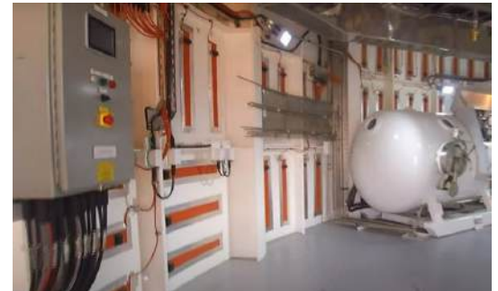
Dive room showing custom SRL-ADJ heating blanket with built-in control
